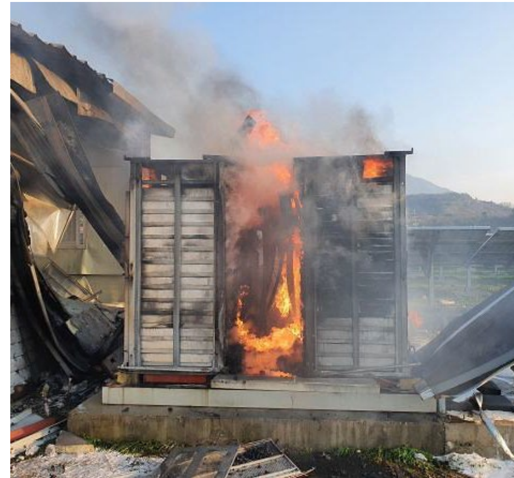
ESS Fire Aftermath Near Seoul, SK, 2021
