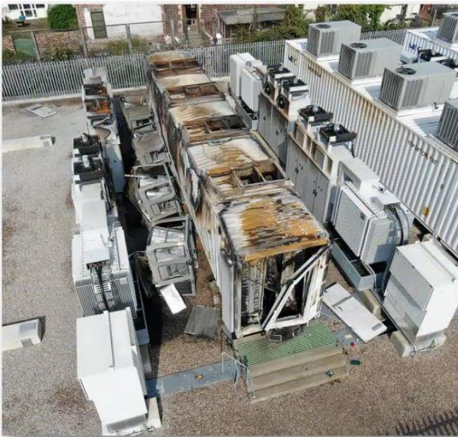
Liverpool, UK, 2020 BESS in container. Battery thermal runaway with explosion.
