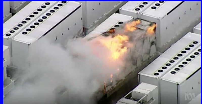
300 MW, Moorabool, Australia, July 2021
